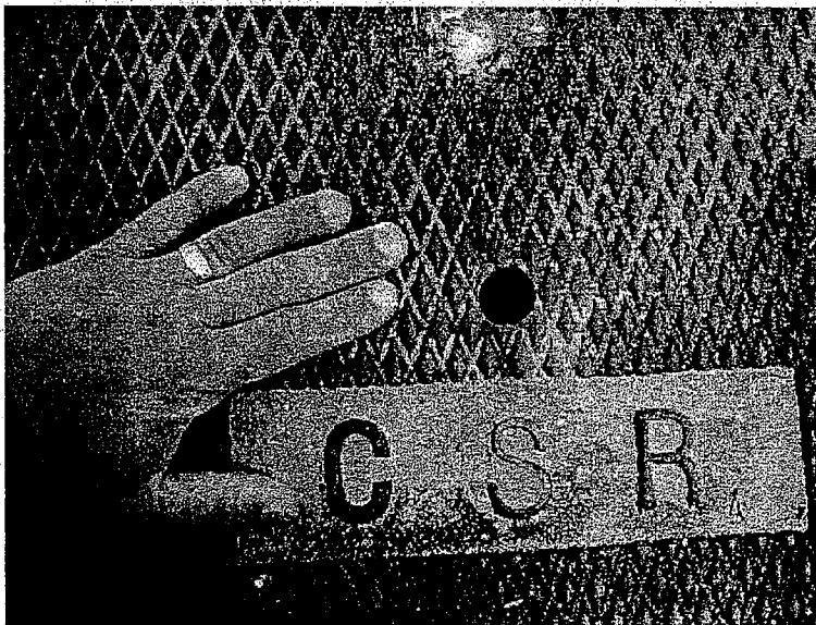
Figure 5. Mosquitoes can access underground sources of water in treatment BMPs from many places, including inlet and outlet pipes, loose-fitting covers, and vent holes. As a general rule, any gap \frac{1}{16} inch (2 mm) or greater is large enough to allow egg-laying females to enter. The hole in this manhole cover is more than large enough to allow mosquito entry. Photo: Marco Metzger.
