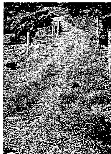
Roads not used in the winter can be "put to bed" for the season. This road has been seeded and will not be used again until the spring. Roads should be properly graded, seeded and mulched, to help prevent erosion. Seeding should occur before October 15 to ensure adequate growth before the winter rains.
